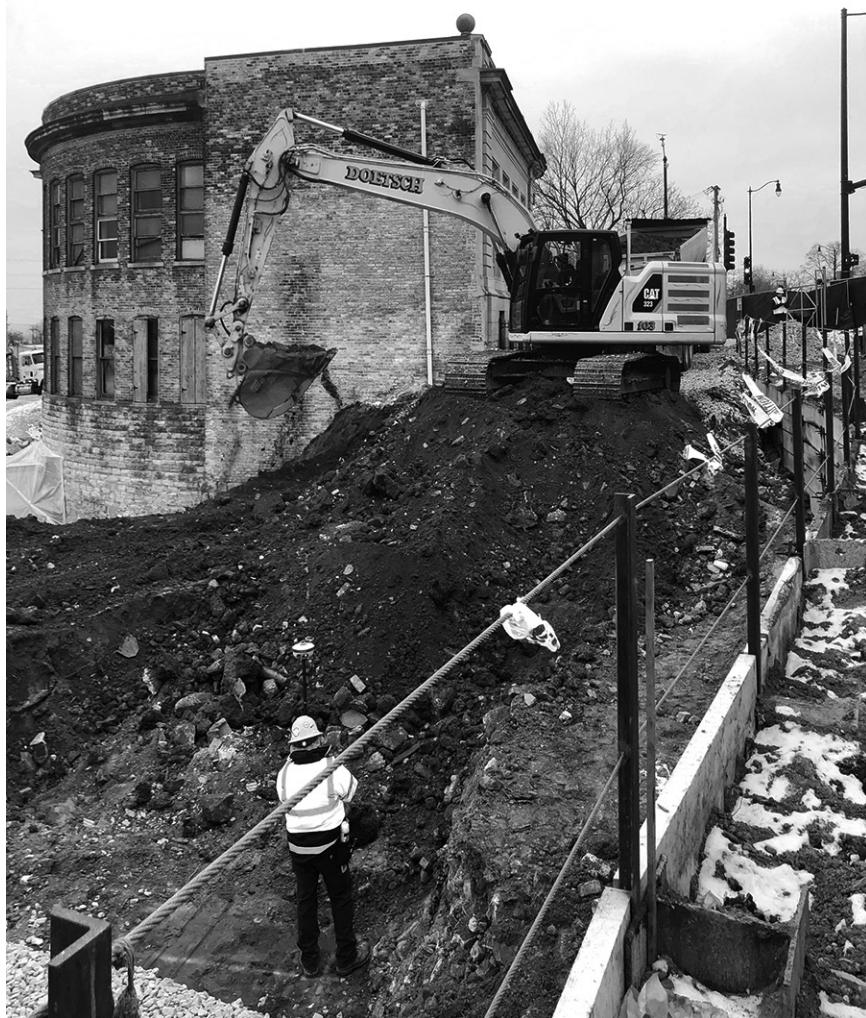
Excavators working on earth retention system in preparation for new addition. Photo courtesy Berglund Construction.
